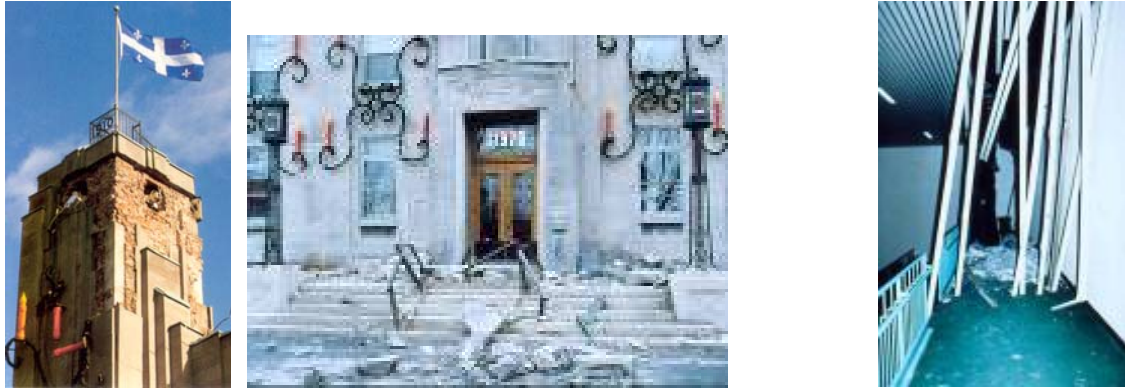
(a) Damage to Montréal East City Hall located 350 km from the epicenter
