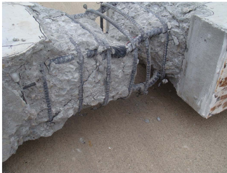
Figure 9. Specimen 9 after testing and after the loose concrete was removed
