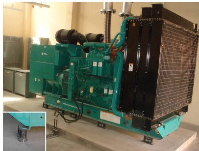
(a) Emergency generator mounted with undersized bolts (H)
