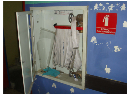
(c) Non-maintained hose-reel cabinet (H&S)
