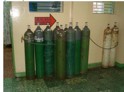
(f) Inadequately secured gas cylinders (H)
