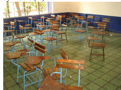
(i) Tables are missing where pupils could hide from falling objects (S)
