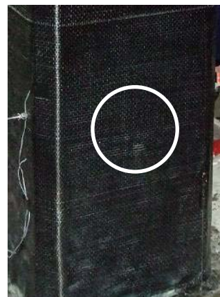
Figure 5. Illustration of the specimen surface after retrofitting.
