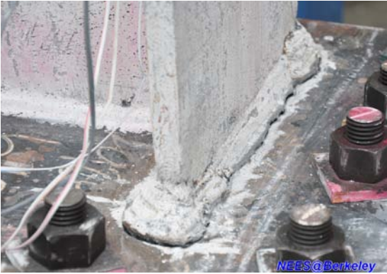
Figure 14. Fracture of the column base flange welding at west side
