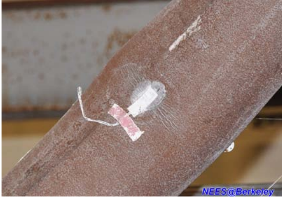
Figure 20. The cracks in the middle of western side of round HSS brace
