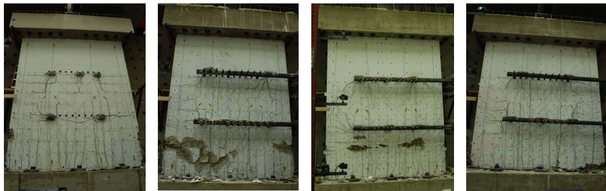
a) PW1 at 1.5% drift b) PW2 at 1.5% drift c) PW2 at 1.25% drift d) PW4 at 1.0% drift Figure 3. Wall specimens at the end of testing
