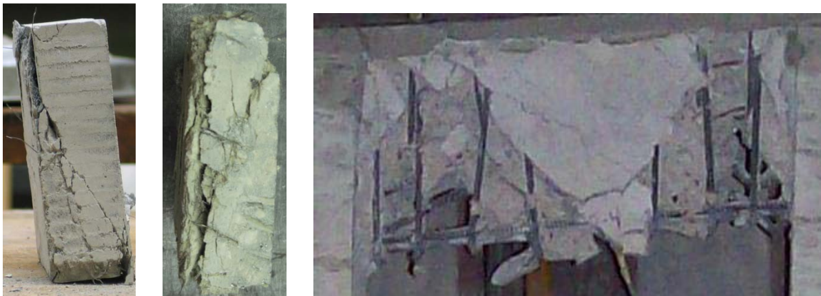
Figure 4. Single shear failure mode (a), and multiple shear failure mode (b), due to biaxial compressive loading; and typical RC coupling beam damage (c).
