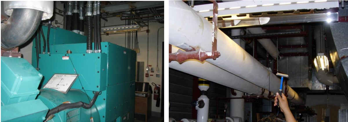
Figure 1. equipment set up and measurement testing at some OFCs.
