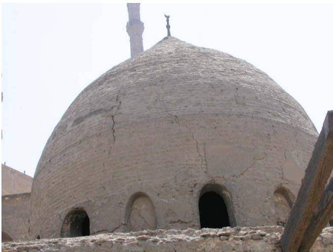
Figure 6. Cracking to domes of Bab El Azab
