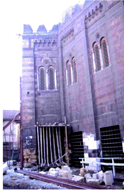
Figure 5. Bulging of external layer of mosque walls Shaykho
