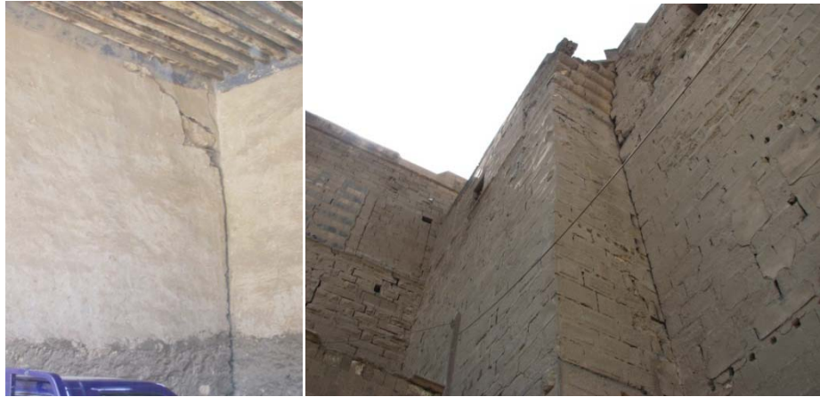
Figure 8. Deep through cracks at corner connection between perpendicular walls (Bab El Azab)
