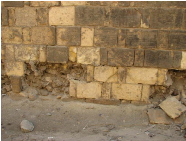
Figure 9. Decay to stones constituting the wall
