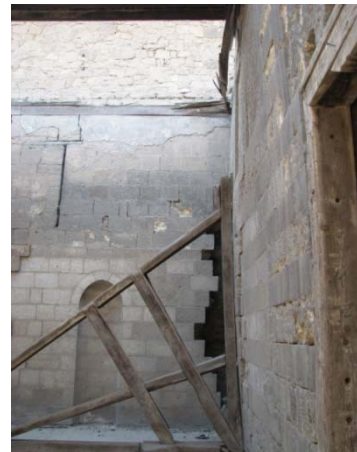
Figure 10. Bulging to wall
