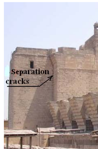
Figure 7. Deep separation cracks
