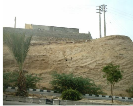
Figure 15. Buildings exposed to landslide
