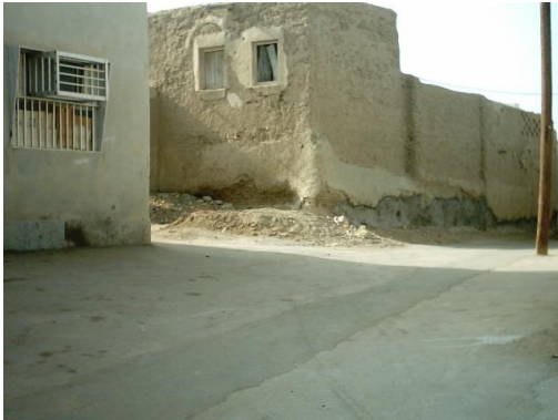
Figure 10. Unreinforced masonry buildings and adobe buildings
