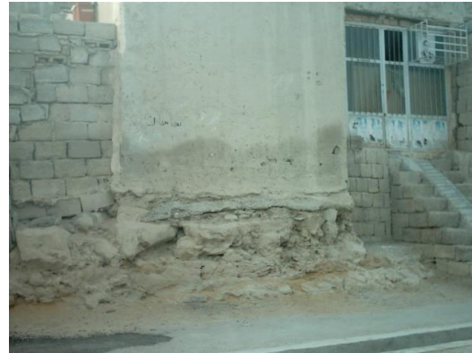
Figure 11. Improper foundation in adobe buildings
