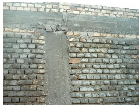
Figure 9. Lack of integrity in concrete ties connection
