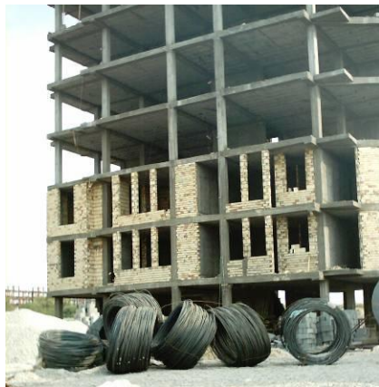
Figure 8. Lack of restrictions of infill and improper portioning of frame elements
