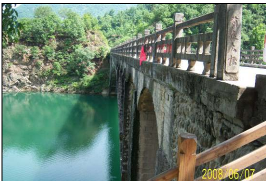
Figure 11. Qian Jin Bridge, a double curved arch bridge with a span length of 75m, was intact
