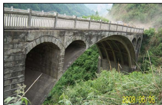
Figure 12. Tong Zi Liang Bridge, a rib bridge with a span length of 30 m, no damage occurred
