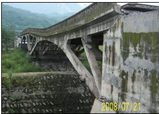
Figure 9. Xiao Yu Dong Bridge collapsed
