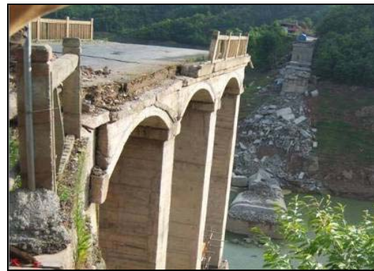
Figure 10. Jing Tian Ba Bridge, a two-span box arch bridge, collapsed
