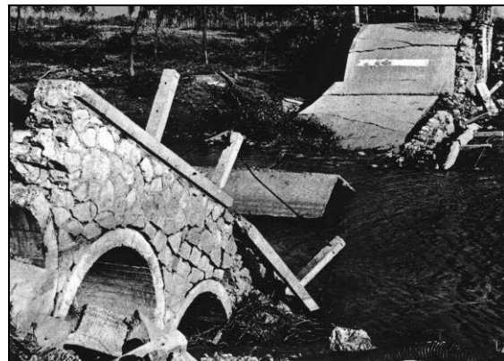
Figure 6. Liu Guan Tun Bridge collapsed
