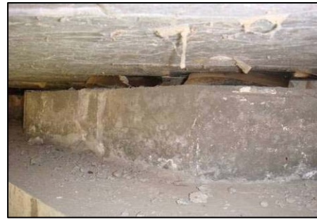
(b) shear failure
