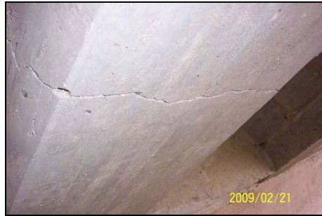
Figure 12. Crack in Arch Ring
