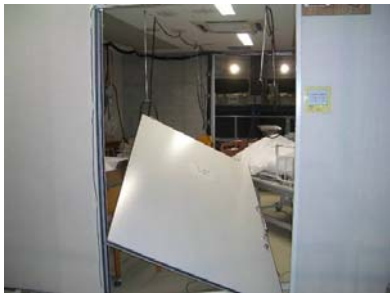
(a-3) Toppled sliding door (Patient room, 4F)
