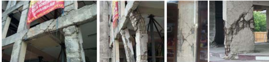
Figure 1. Damage patterns in old type RC members.
