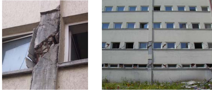
Figure 6. Captive column effect and buckling of longitudinal steel
