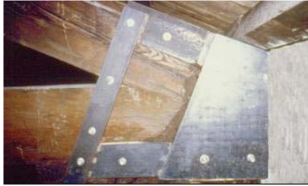
Figure 3. Intervention producing overstrengthening on the rafter to tie-beam node.
