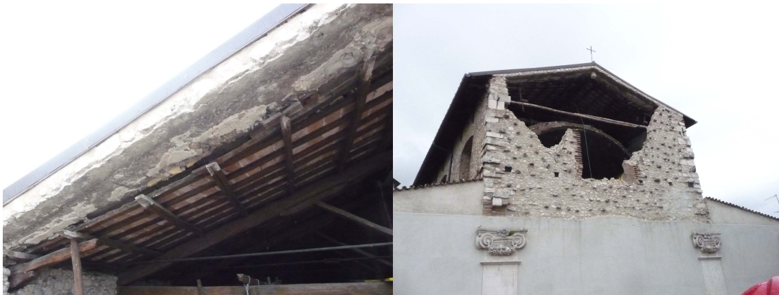
Figure 7. Increased dead load on roof structure (left), church of S. Biagio Amiterno, L'Aquila.
