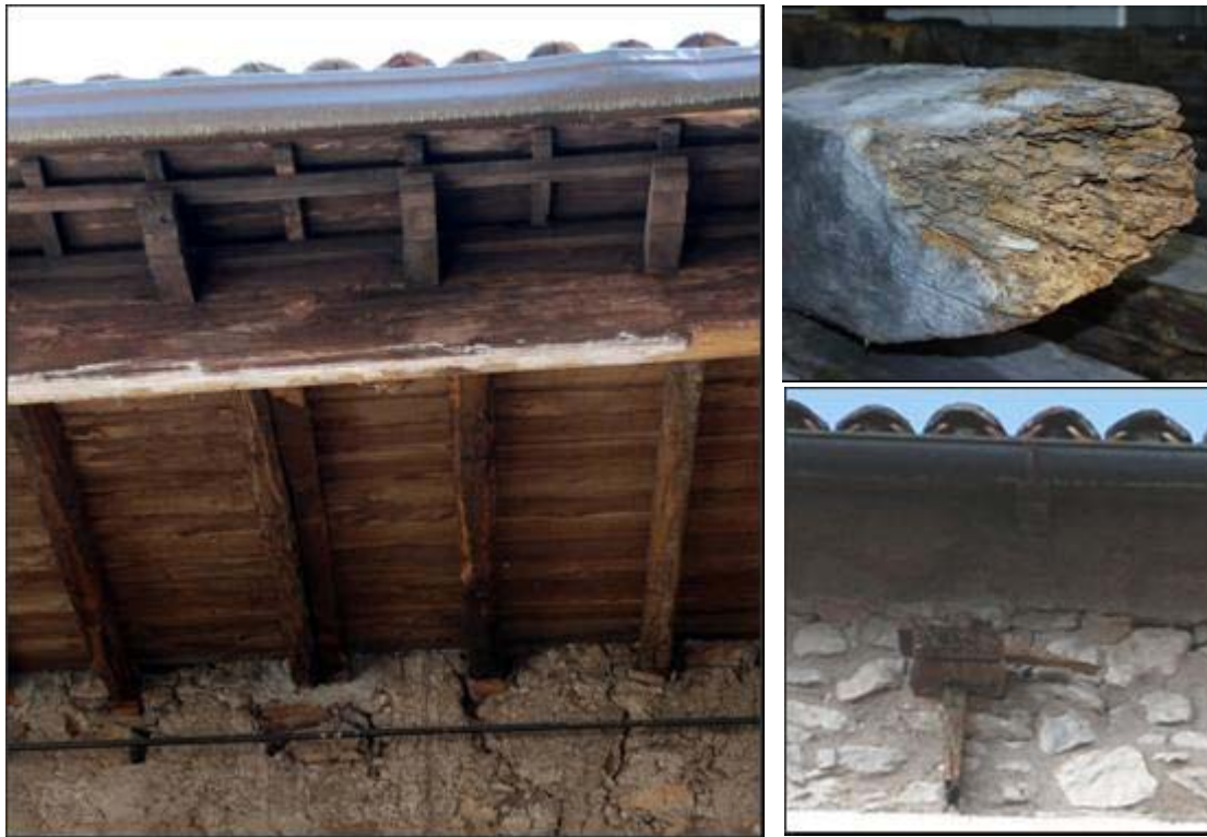
Figure 5. Different support conditions; built-in elements (left); decayed built-in beam end (top right); an old-time external restraint maintained support of the timber truss in the L'Aquila earthquake (bottom right).
