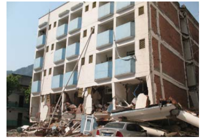
Figure 3. Soft story collapse
