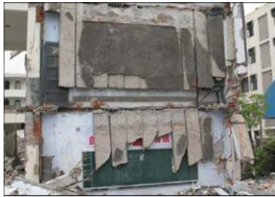
Figure 1. Collapsed ceiling/floor planks
