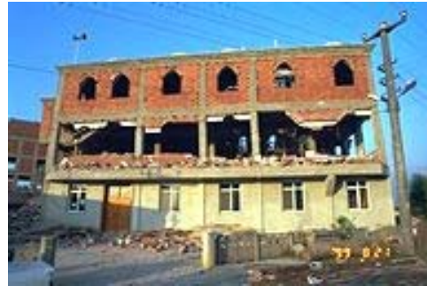
Figure 6. URM infill collapse (NISEE 2009)
