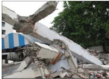
Figure 2. Collapsed concrete beam
