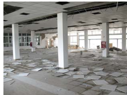
Figure 2. Partially collapsed ceiling, Sichuan Earthquake (M8.0, 2008).
